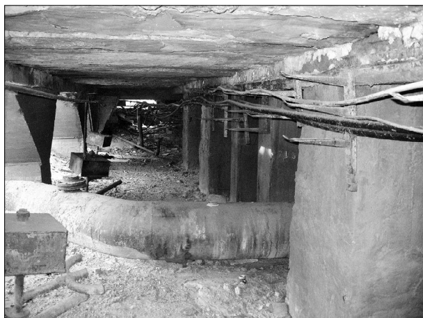
Fig. 1. Ventilated space under the main building of the Yakutsk Combined Heat and Power Plant. (A photo by S.I. Zabolotnik, 05.11.2009).
