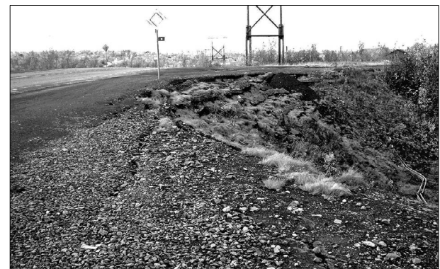
Fig. 5. Stepwise detachment of slopes and embankment top.
