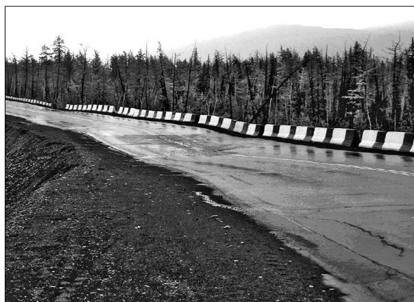
Fig. 3. Local carriage way settlement within a segment of a broken drainage pipe.
