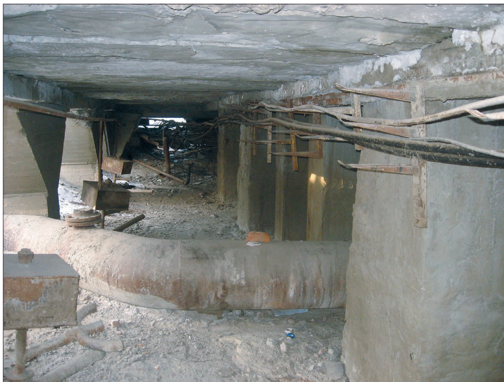
Fig. 6. The cross ventilated basement under the main building of the Yakutsk CHPP.
