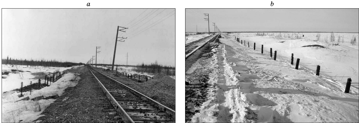
Fig. 18. System of long thermosyphons after installation (a) and in winter season (b).
