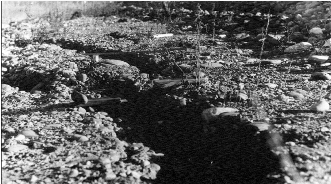
Fig. 4. Vector of motion of embankment surface in its different parts in seasonal (autumn–spring) cycles for three years (a) and cracks on the sides (b).
